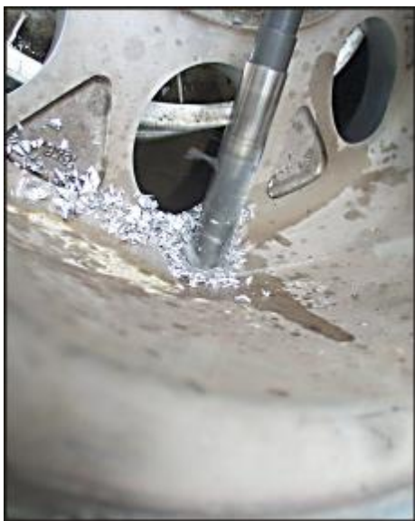
Figure 6 Measure twice, hold your breath, then drill the hole precisely where you want it. For inside stems, remember to inspect for brake drum, caliper and other items that may interfere with free rotation.
